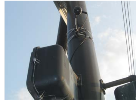
Pedestrian detection sensor (FLIR™) installed at the SR 13 and Haley Road Intersection in 2015.
