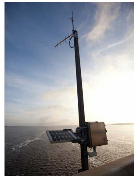
One of the Road Weather Information System (RWIS) devices installed on all 22 bridges over waterways. The street flood warning sensors will be integrated to provide water stages and predict street flooding in downtown Jacksonville.
