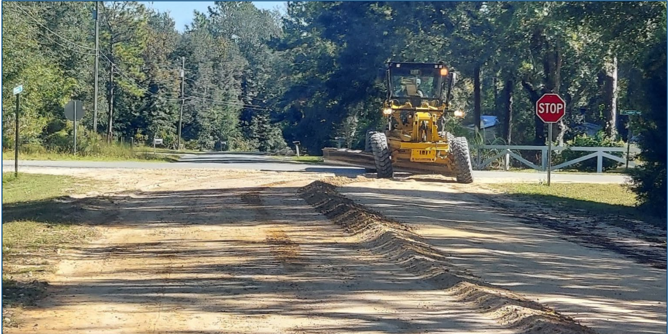
A Clay County crew grades Chicory St, which is considered a difficult to maintain road.
