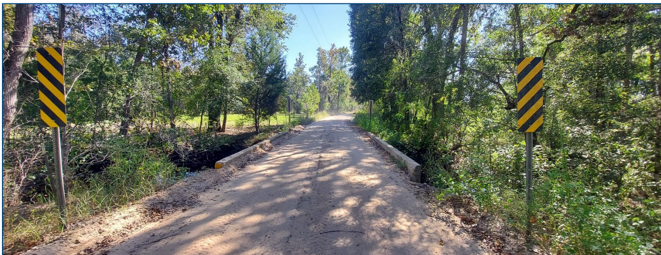
Prior to paving Sweet Moody Rd, the bridge over Greens Creek will need to be replaced.
