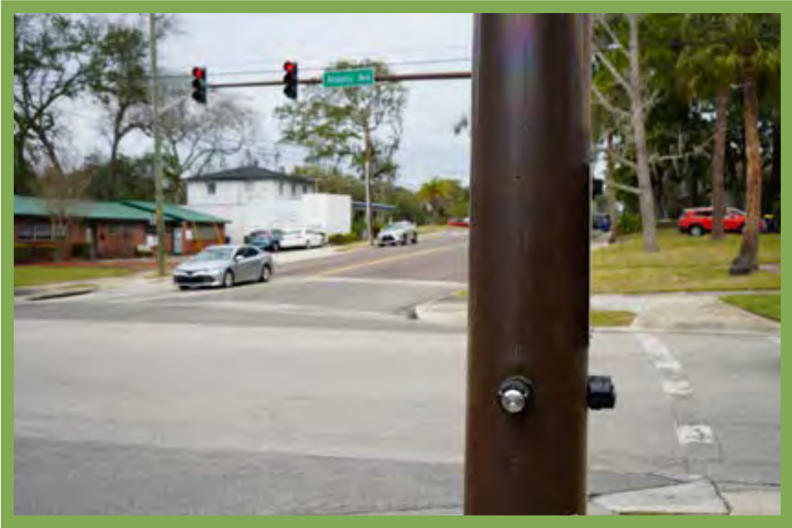
Missing signage at the pedestrian push button (at the southeast corner)
