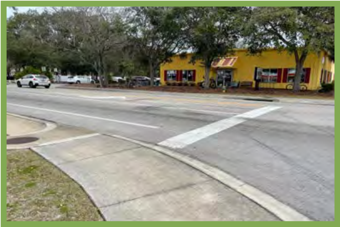
North crosswalk is not marked (looking toward the northeast corner)
