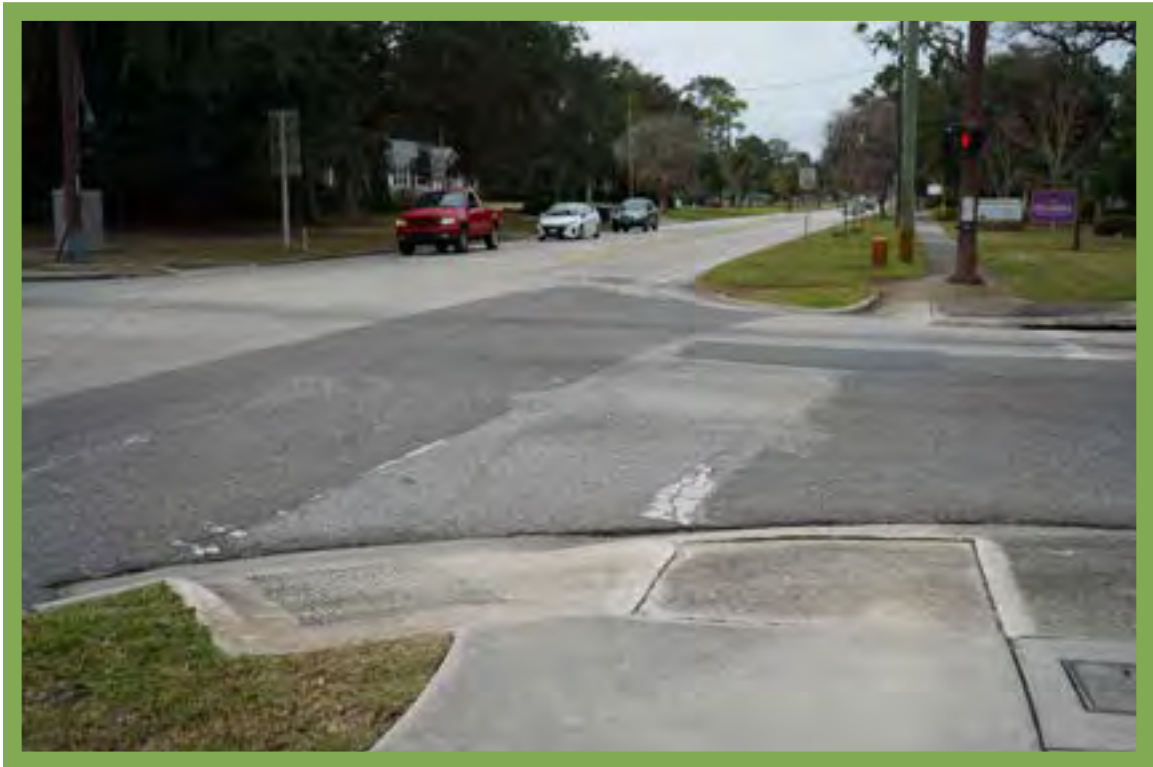
North crosswalk is not marked (westbound)
