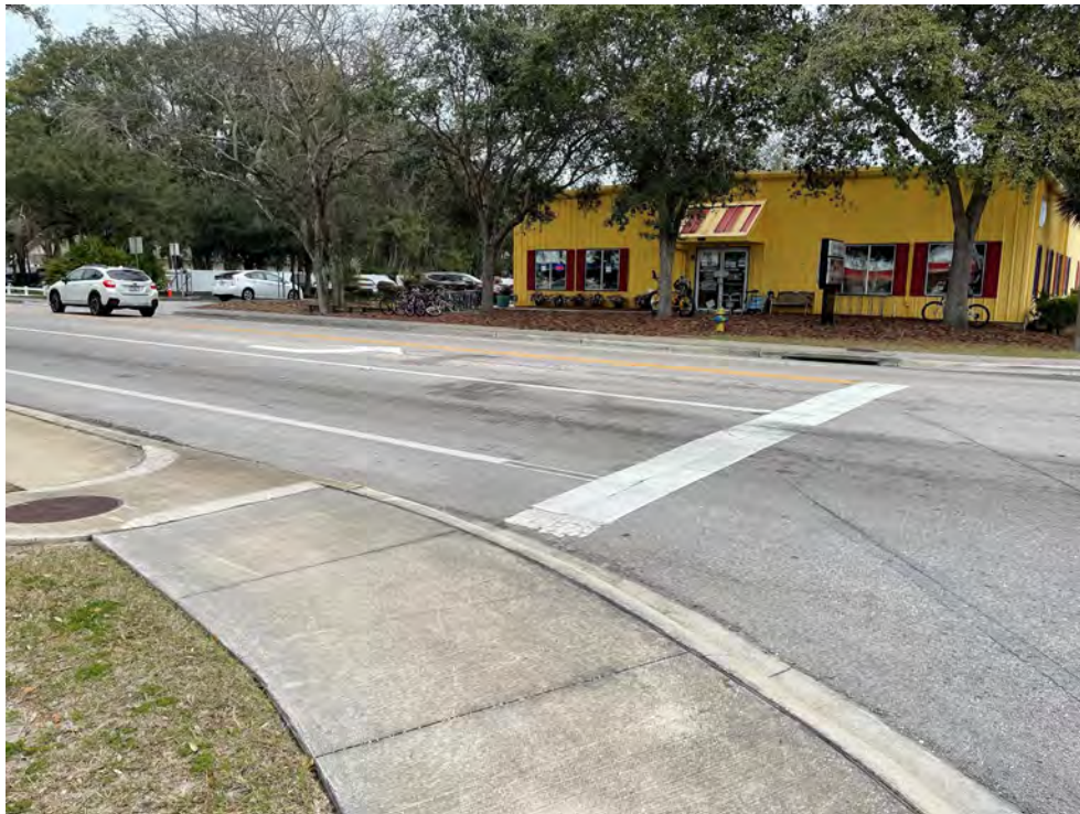
Photo: The northern crosswalk is missing at the 14 th Street and Jasmine Street intersection (north side of the intersection)
