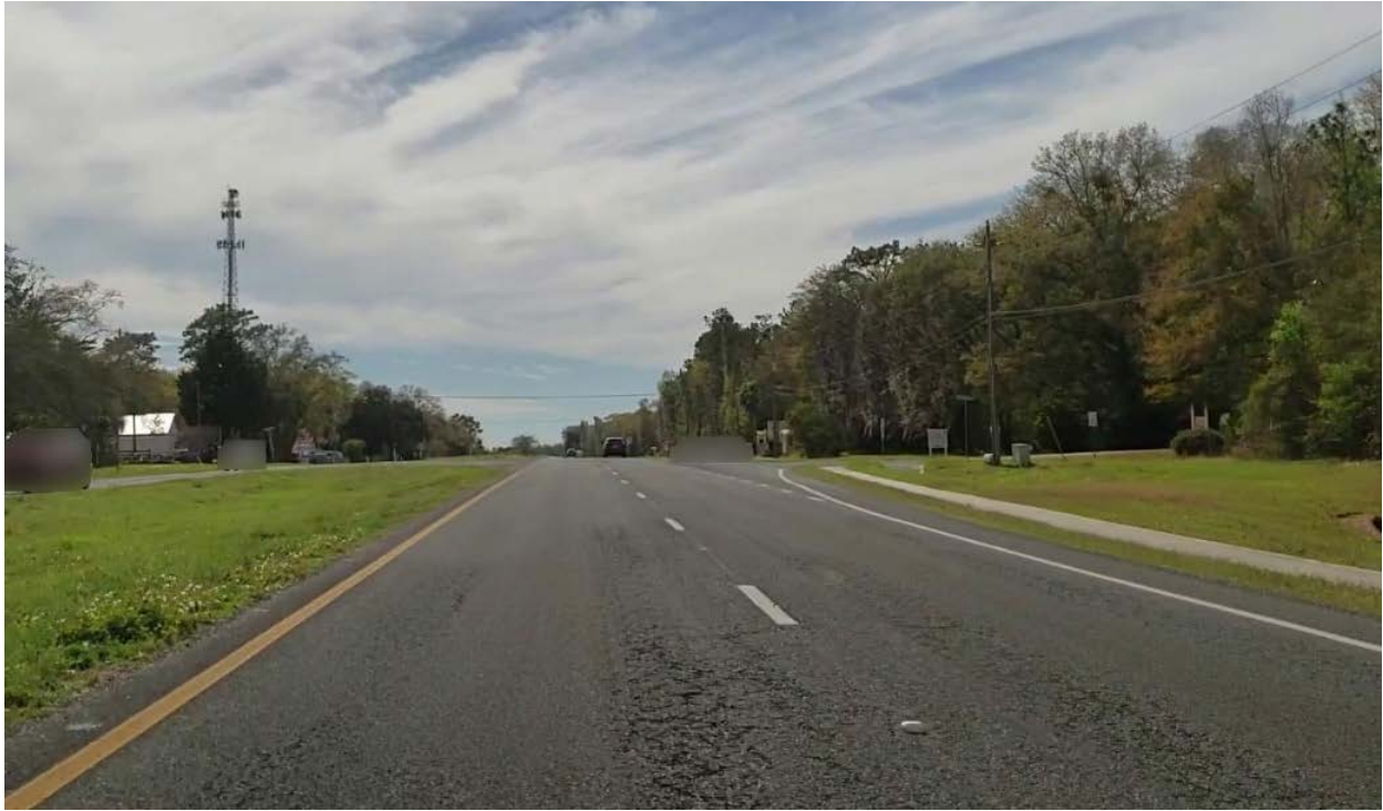
Figure 14. Raveling Near Peppergrass Street in the Southbound Lanes
