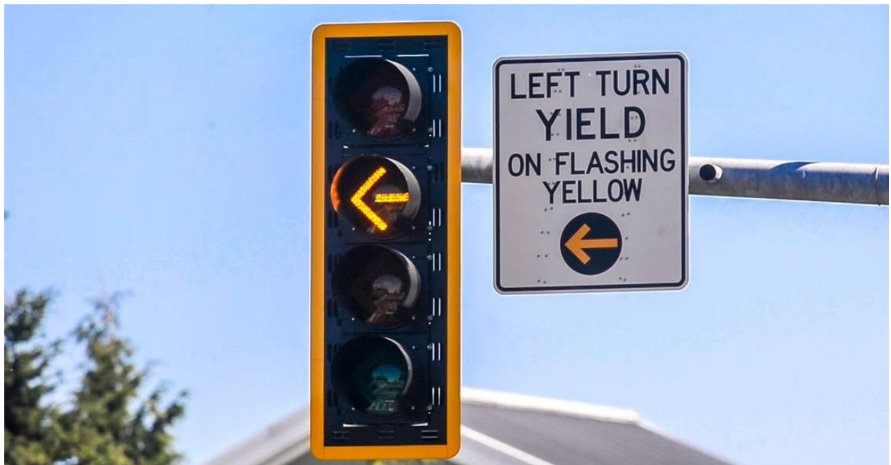
Figure 28: Flashing Yellow Left Turn Arrow with Yellow Retroreflective Backplate
