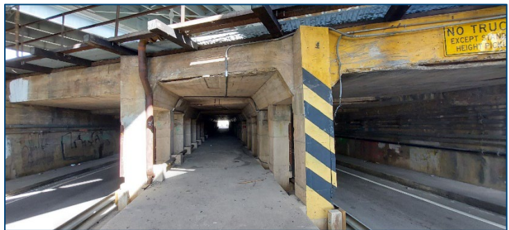
The “subway” provides a connection under I-95 on Myrtle Avenue between Dennis Street and West Bay Street.
