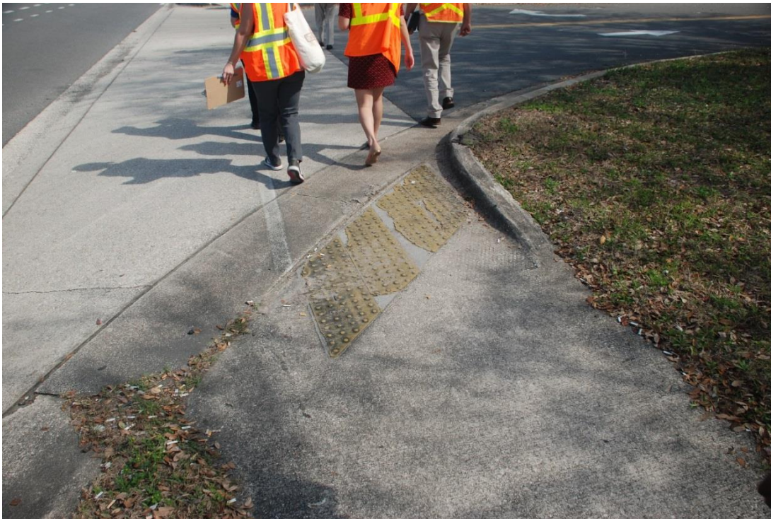
Detectable Warning Surface that needs replacing (east of St. Johns Bluff Road near Walgreens)
