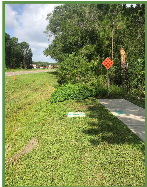
Sidewalk Gap on Dobbs Road Cutoff east of SR 207 (Gap ID 223)
