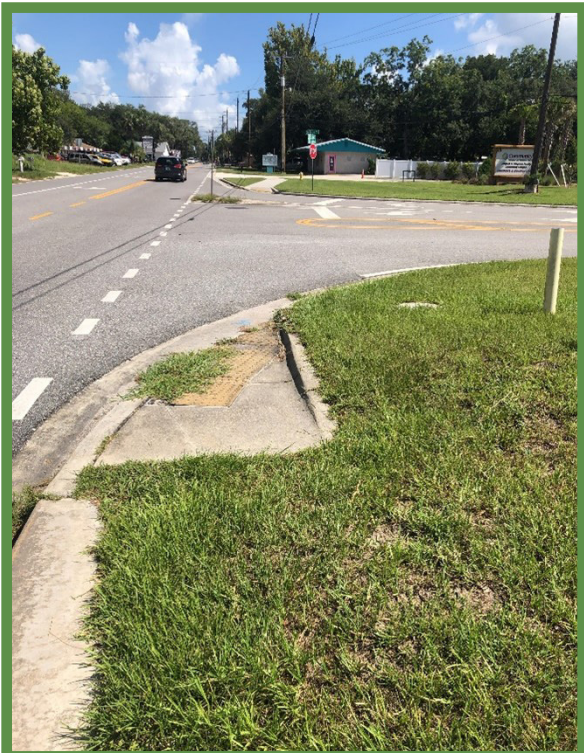
Sidewalk Gap at Old Dixie Hwy. and Old Moultrie Road (Gap ID 203)
