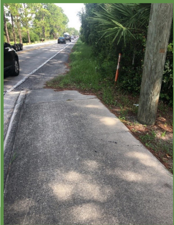
Sidewalk Gap on South Holmes Boulevard northwest of SR 207 (Gap ID 201)
