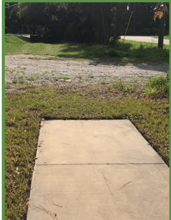
Sidewalk Gap on Dobbs Road Cutoff west of Dobbs Road (Gap ID 225)
