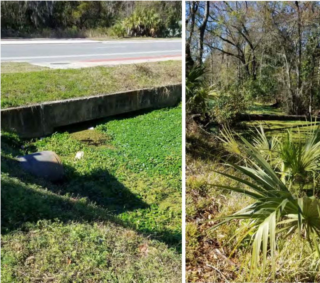
View of US 301 culvert outfall. The water surface elevation in the downstream channel is near the culvert top during a dry period. Note the aquatic vegetation growing on the water surface.
