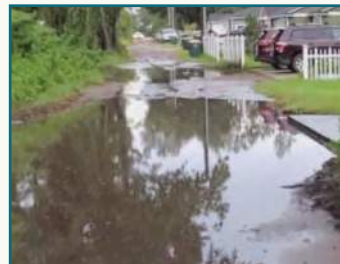
Flooding/ponded water in road
