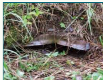
Clogged/crushed storm culvert under road
