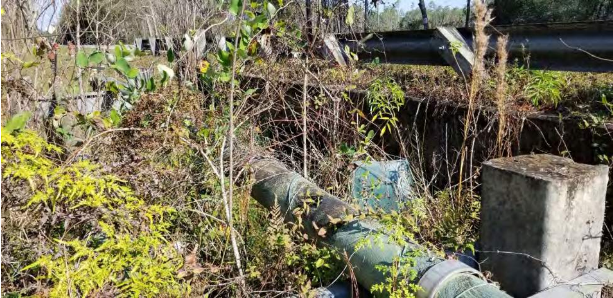
Existing culvert under Yellow Water Road with a view of downstream culvert channel conditions.
